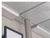
Penetrated down pipe
